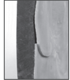
XLPE with linear liner (delamination example)
