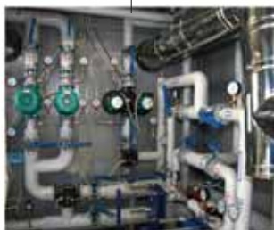
Industrial water treatment systems
