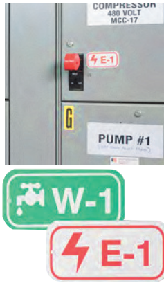
Step 3: Identify and mark all energy control points
